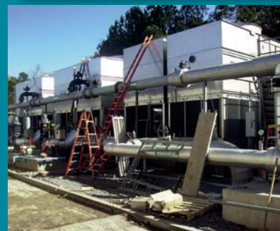
Telecommunications Company 18.5 MW
