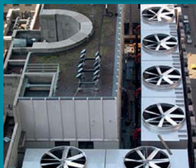
HVAC for Skyscraper 35.7 MW
